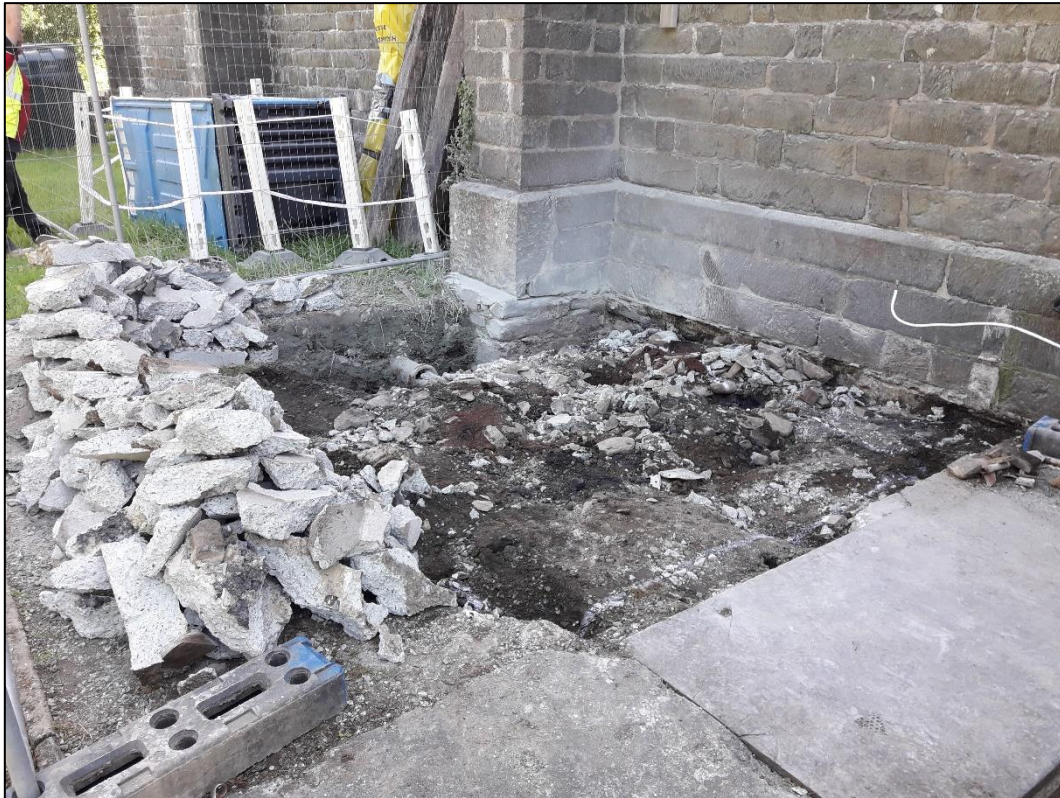
Photograph 9 – Concrete pad broken out to allow the underlying soils to be assessed (28.07.20)
