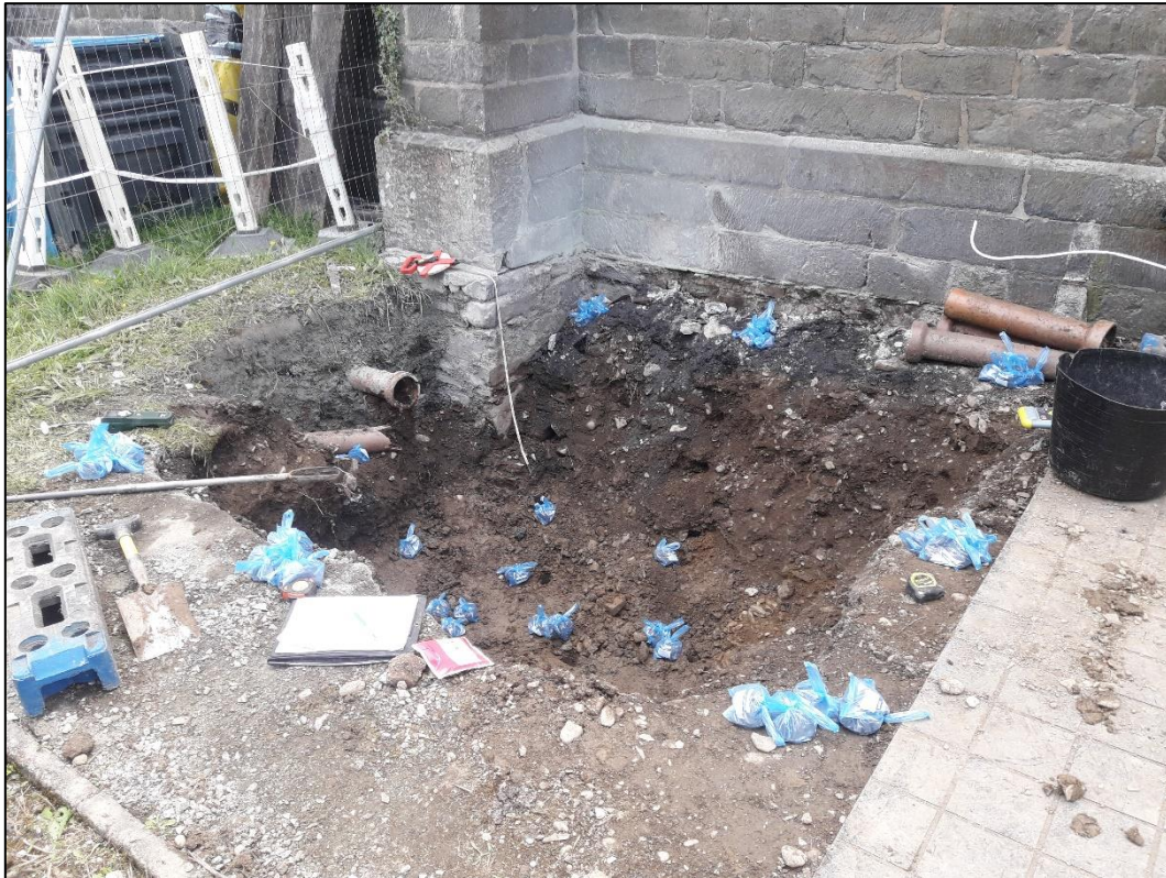
Photograph 11 - Soils were excavated over a 2.7m x 2.3m area to a maximum depth of 1.2m (30.07.20)
