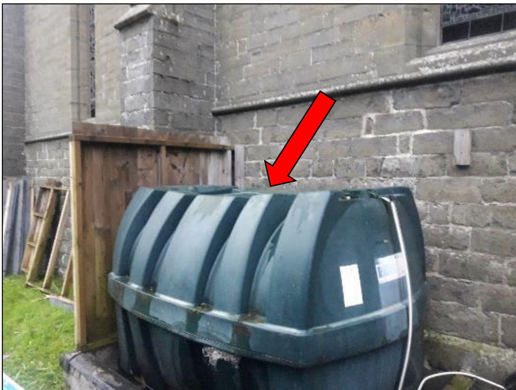
Photograph 3 – The OST was bowed in its centre and bulging close to the crack (18.06.20)
