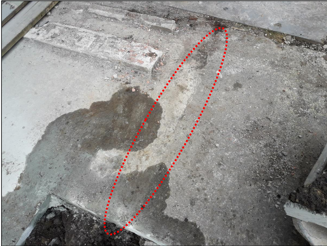
Photograph 5 – Crack in the concrete pad allowed migration of kerosene to underlying soils (28.07.20)
