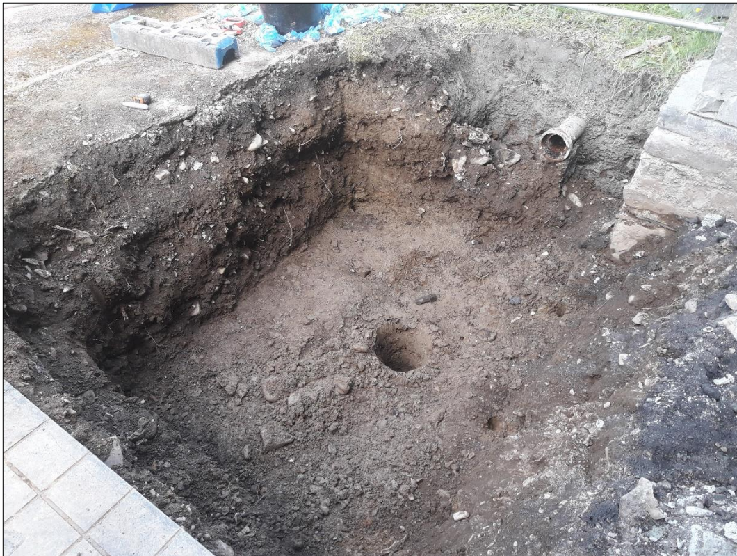
Photograph 6 – Extent of excavation beneath the concrete pad (30.07.20)
