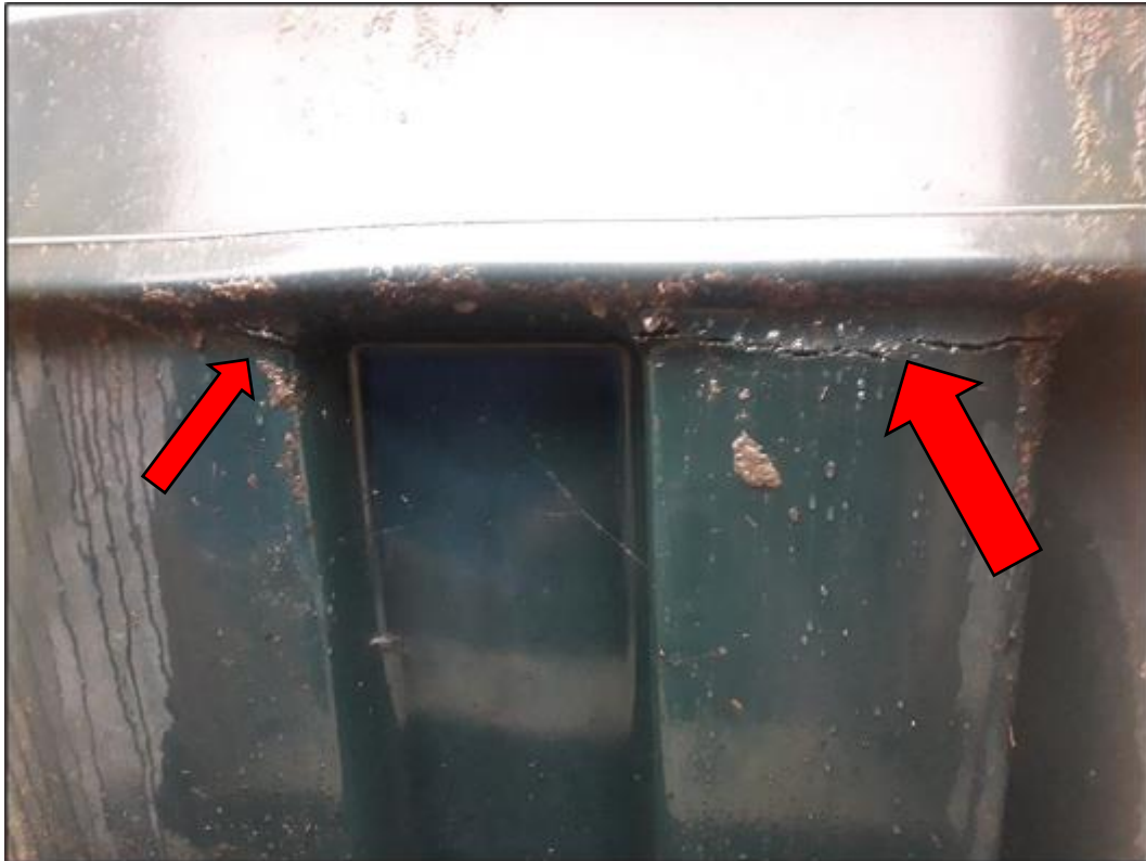
Photograph 2 – Fence panels removed to reveal a large crack and smaller cracks in OST (18.06.20)
